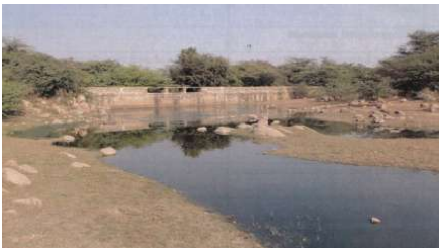
Figure A3.3 Check dam on JNU campus, New Delhi.
