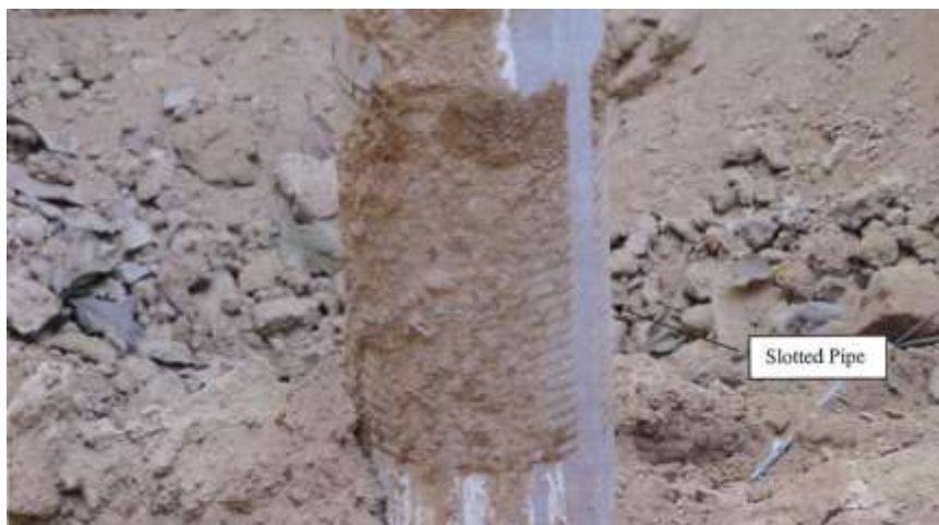
Figure A3.1 Recharge well with slotted pipe in porous media filter after excavation for de-silting and installation of geo-textile around the slots.
