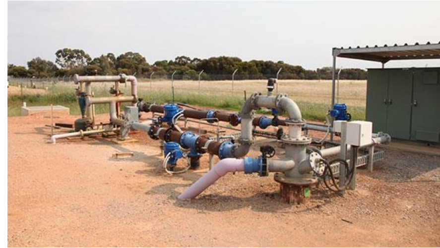
Infiltration wells in Salisbury, Australia
